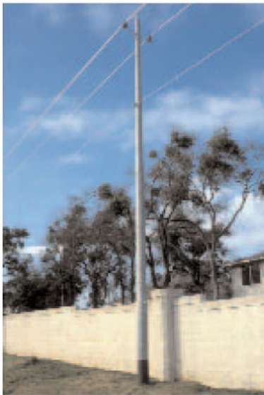
Today, 90 percent of all new major power distribution projects at Austin Energy include steel poles.
