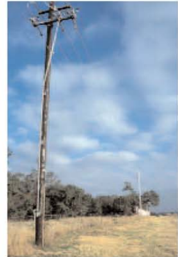
Austin Energy has found the weathering steel poles are ideal as replacement poles in established neighborhoods, as the pole "blends right in to the existing line."
