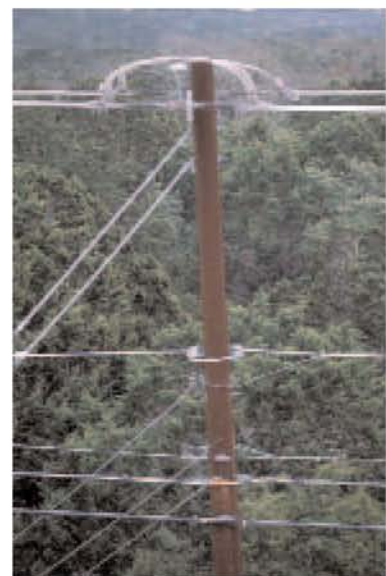
Pictured here is a 765 AAC double dead-end pole on a 50LD2 weathering steel pole with downguys, set in Austin's hilly terrain.
